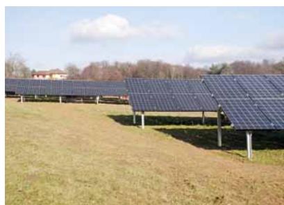
The largest freestanding system in the region: This solar plant in north-slovenian Gornji Petrovci has a power output of 81 kilowatts.
