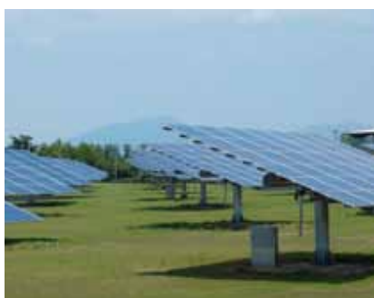
The largest tracking system in Lombardy: 92 racks direct the solar modules toward the sun.
