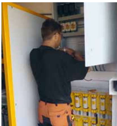
Grid support: The SolarMax inverters do not switch off when there are brief grid malfunctions. Here is a Solea employee at a DC fuse cabinet.
