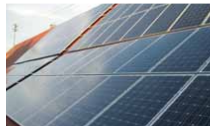
Good yields despite partial shadowing: Sputnik’s MT series works at the maximum power point of the solar generator even in difficult conditions, as does this 25-kilowatt test plant of Actensys GmbH in Waldstetten.
